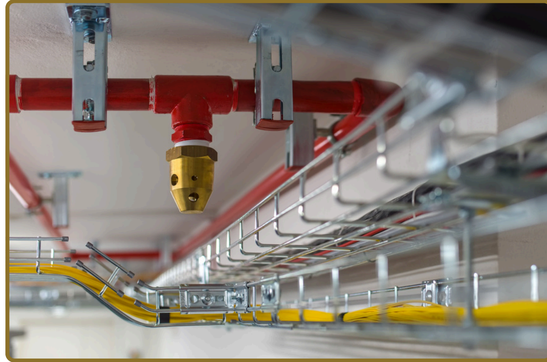
Fire Suppression System
